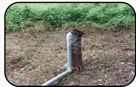
Use of unused borewells for groundwater recharge
